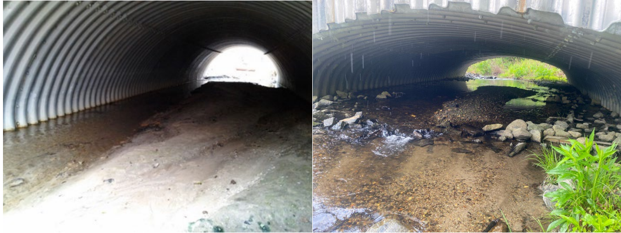
Figures 2 and 3. Wide corrugated metal pipe (Wayne County, SR 1300, Unnamed Tributary) retaining bedload (left) and aluminum box culvert (Transylvania County, #870163, North Prong Glade Creek) with notched sills and baffles buried by bedload (right, note partially exposed sill in photo right).
