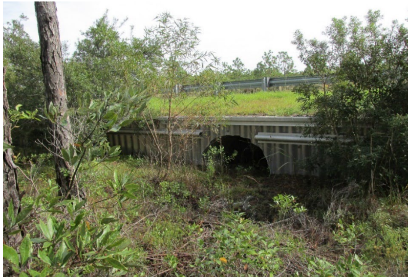
Figure 17. Culvert designed for small and medium animal passage on EF Middleton Blvd. Brunswick County.
